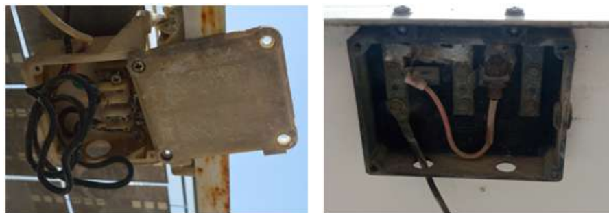
Fig. 6.11: Examples of damaged junction boxes observed during the survey in old modules.
