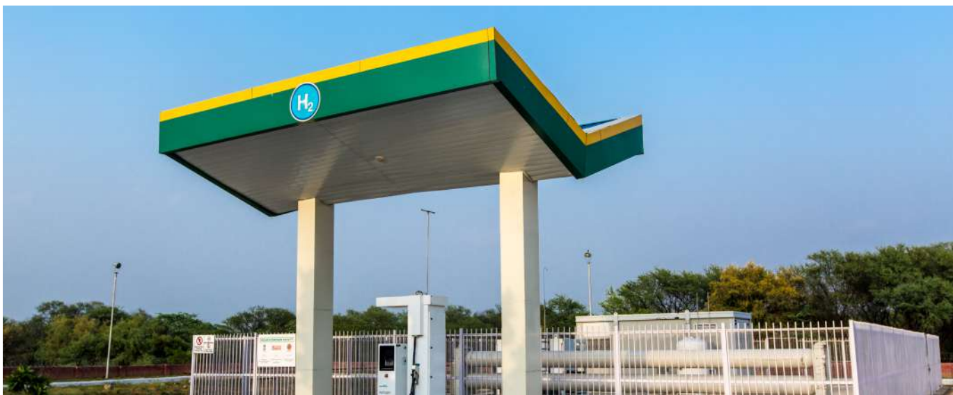
Figure 6.1 Hydrogen Production cum Dispensing Facility at NISE
