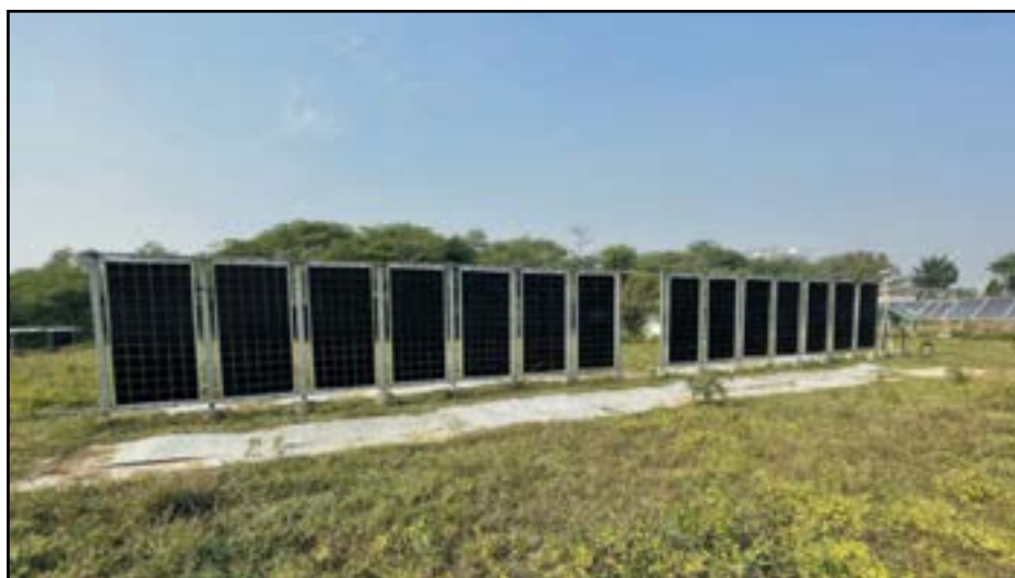
Figure 3.6: Bifacial solar PV modules at vertical tilt (5 kWp)
