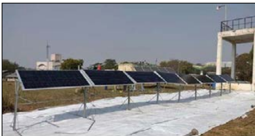
Figure 3.16: Solar Water Pump Test Setup using Bifacial Module
