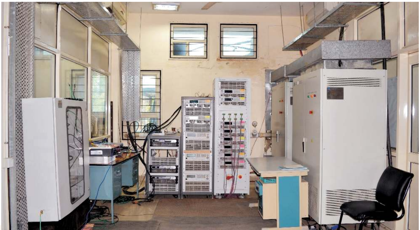
Figure 3.5: Power Electronics Laboratory Setup
