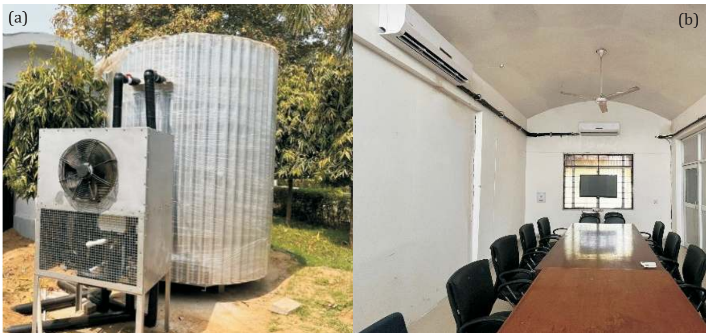
Figure 2.9: Photograph of (a) heat pump outdoor unit with thermal storage tank and (b) indoor unit of heat pump
