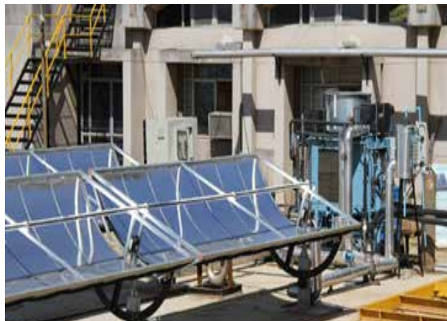
Figure 4.4: 15 kW Solar Absorption Refrigeration System (Air Cooled)
