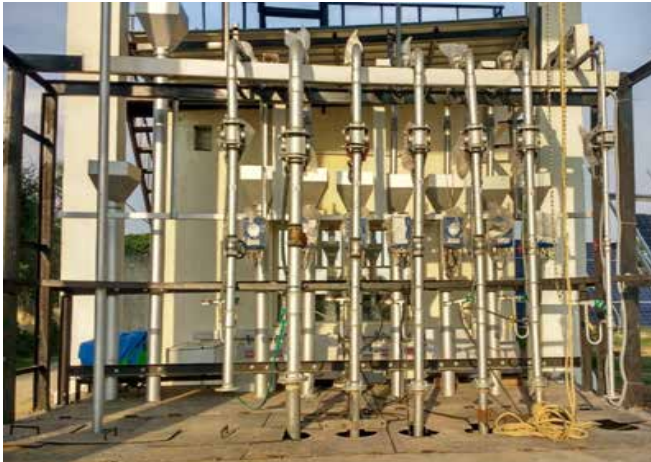
Flow and pressure measurement and control arrangement for pump testing at test bed
