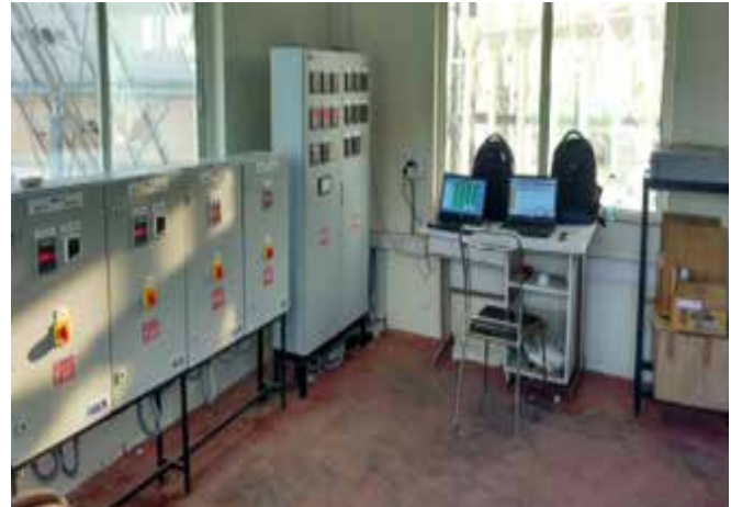
Control room for display and data logging
