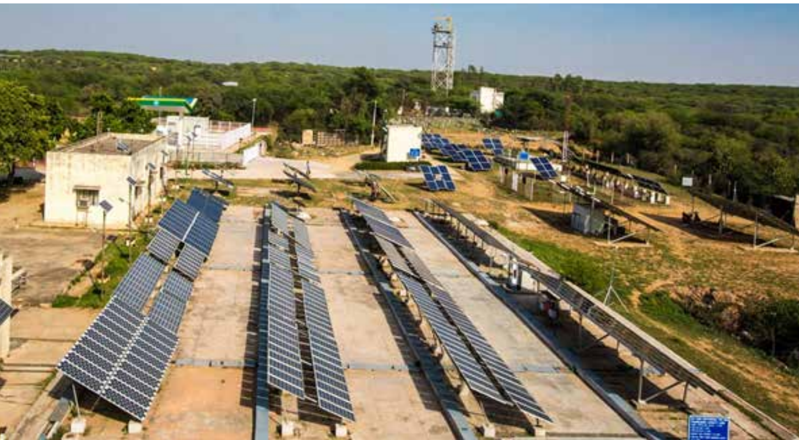
Solar PV Outdoor Test Bed Facility showcasing different technologies
