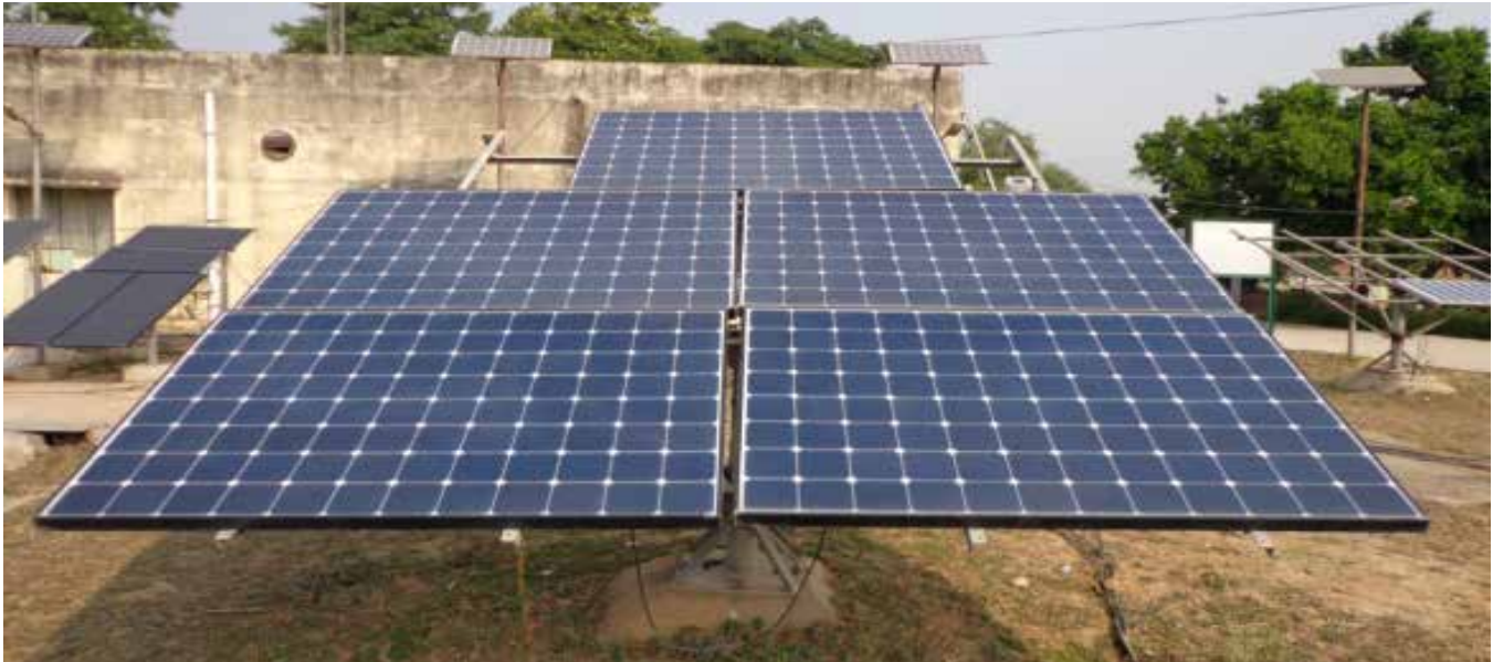
Test set up for Sun power technology PV module
