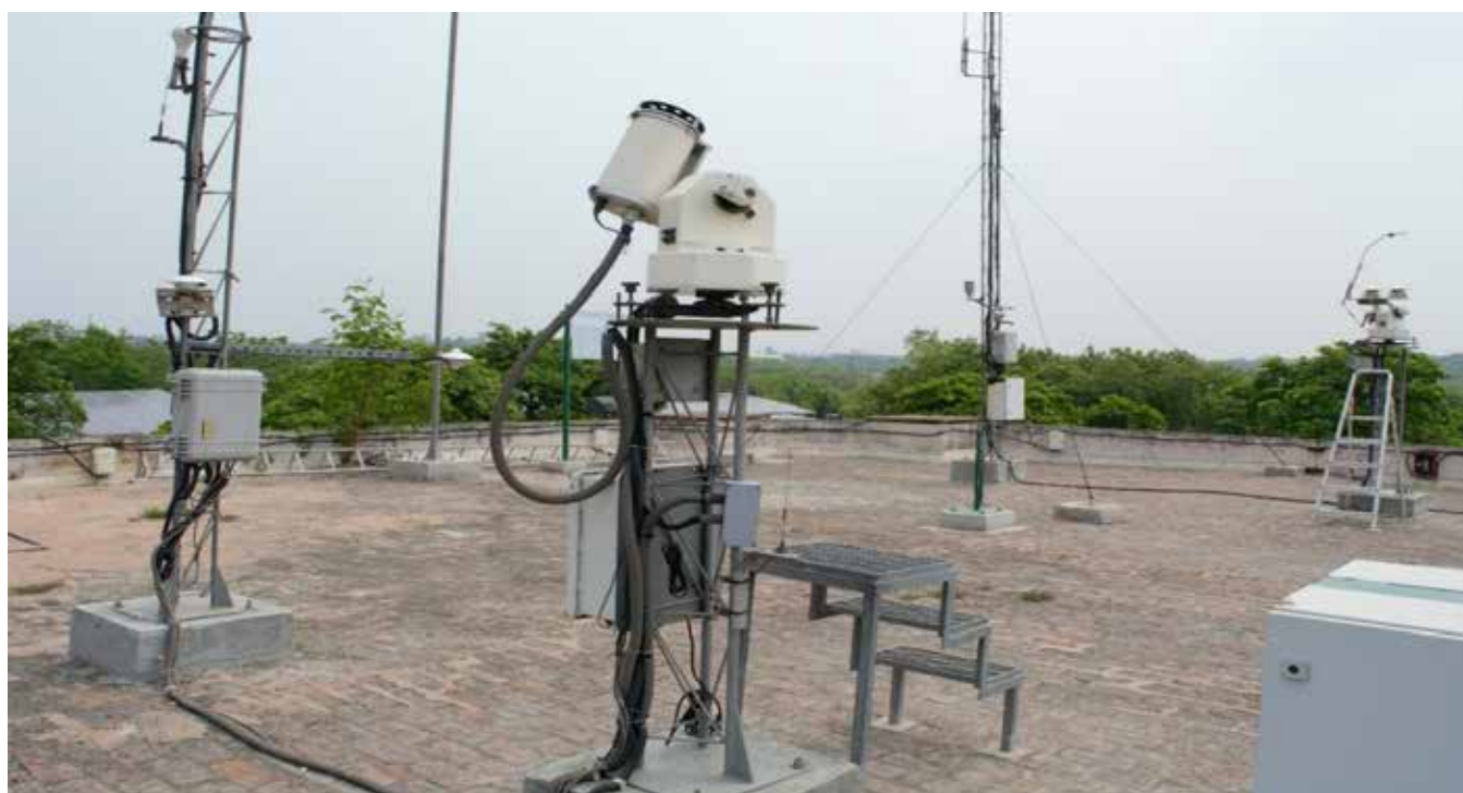
Figure 3.1 : SRRA facility at Aditya Bhawan rooftop in NISE
