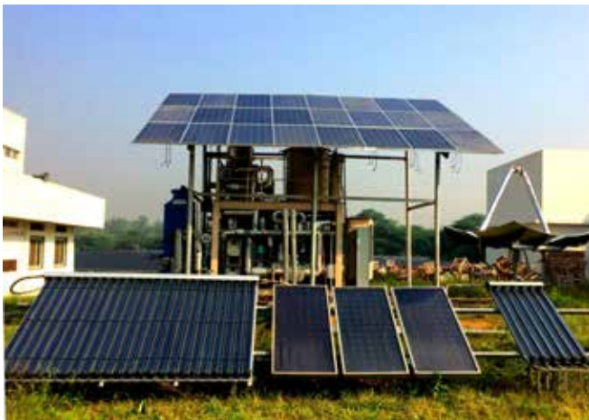
Figure 5.11 : Test facility for testing of hot water/steam-based CST systems
