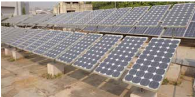
Figure 4.16 : Test set up for Mono C-Si technology PV module
