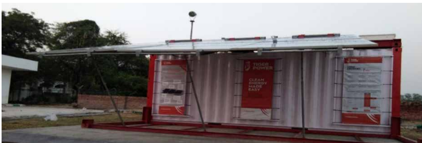
Figure 7.3 : Hybrid System installed in NISE by M/s Tiger Power, Belgium under a collaborative project
