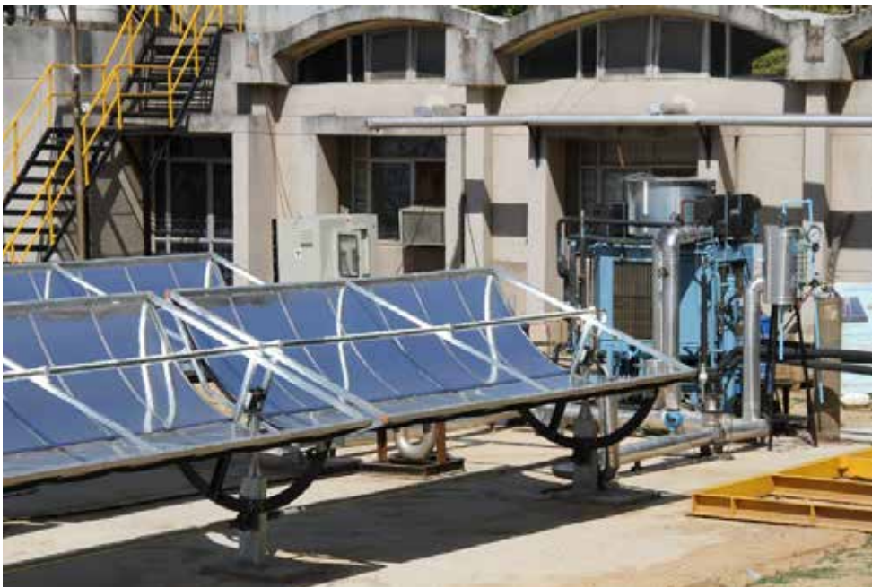
Figure 5.6: 15 kW Solar Absorption Refrigeration System (Air Cooled)
