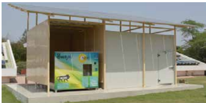
Figure 6.9: Prototype RO system installed at NISE
