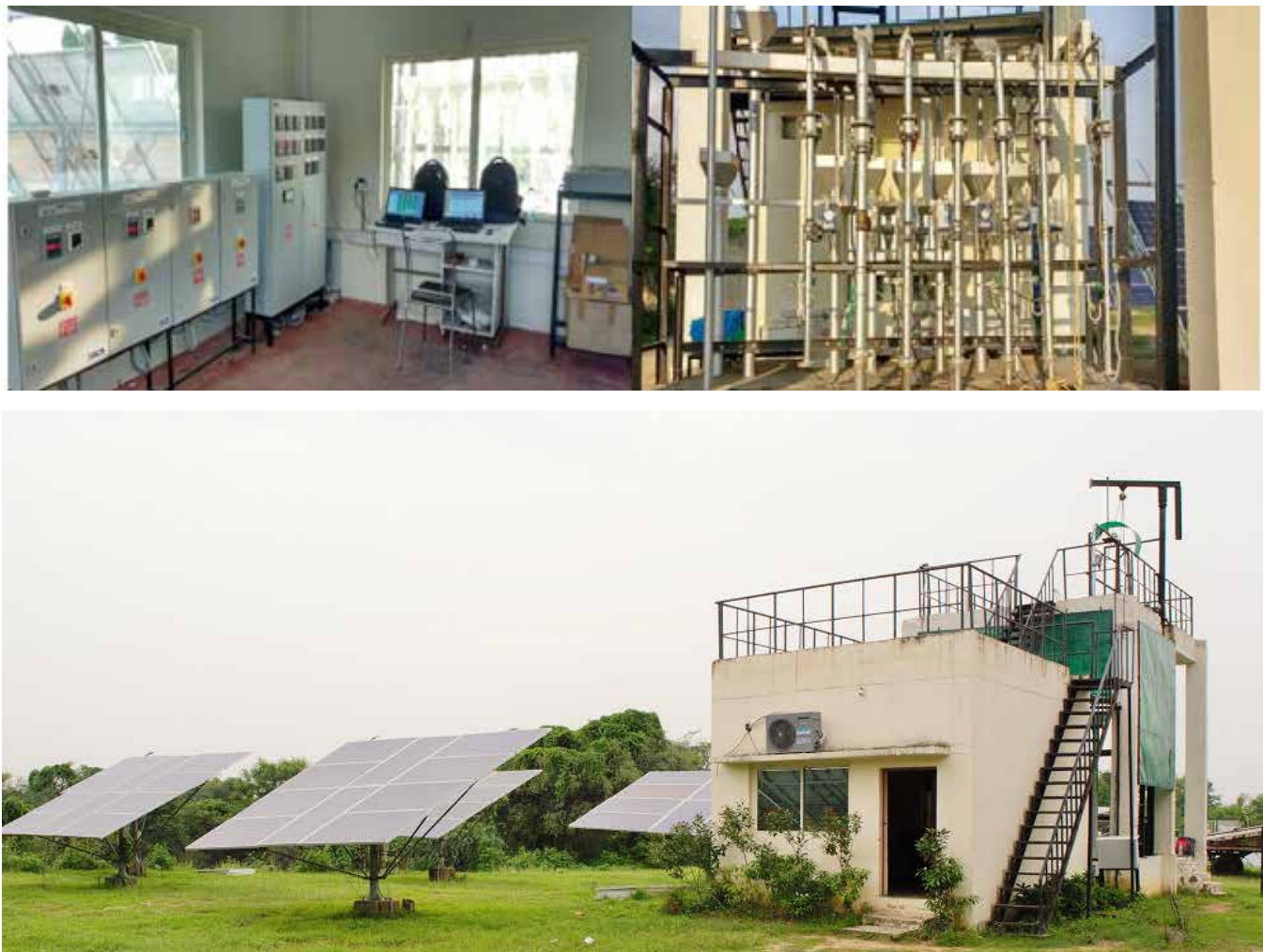
Figure 4.8: Pump testing arrangement at test bed along with Control room for display and data logging
