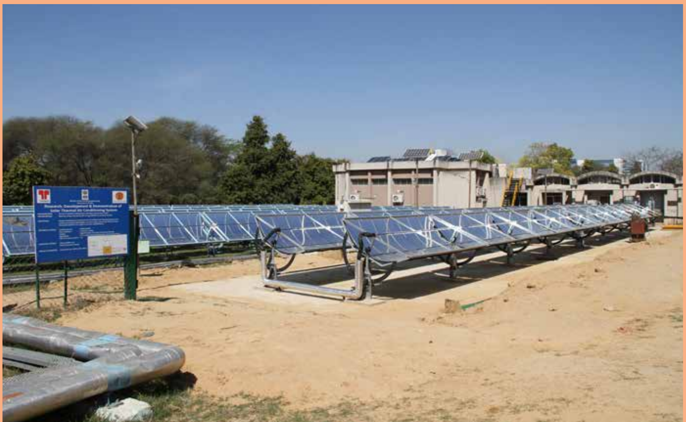
Solar Thermal Air Conditioning System at NISE
