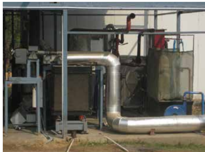
Figure 5.10 : Experimental setup of 50 kW Solar Biomass Hybrid Cold Storage Cum Power Generation System for Rural Electrification
