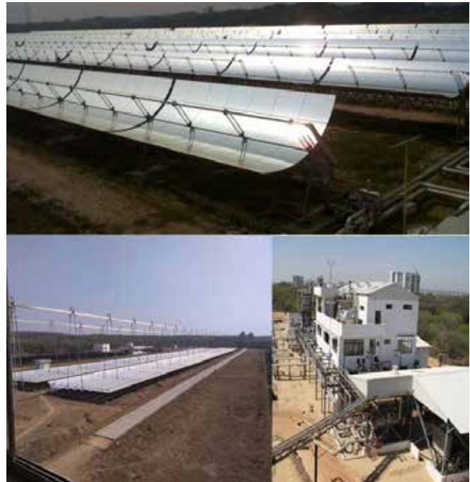
Figure 5.1 : 1 MW Solar Thermal Power Plant at National Institute of Solar Energy
