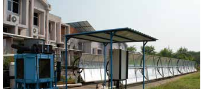
Figure 5.3: 15 kW double effect vapour absorption system
