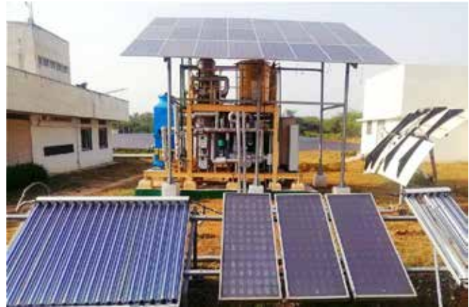
Figure 5.6: Test facility for testing of hot water/steam based CST systems
