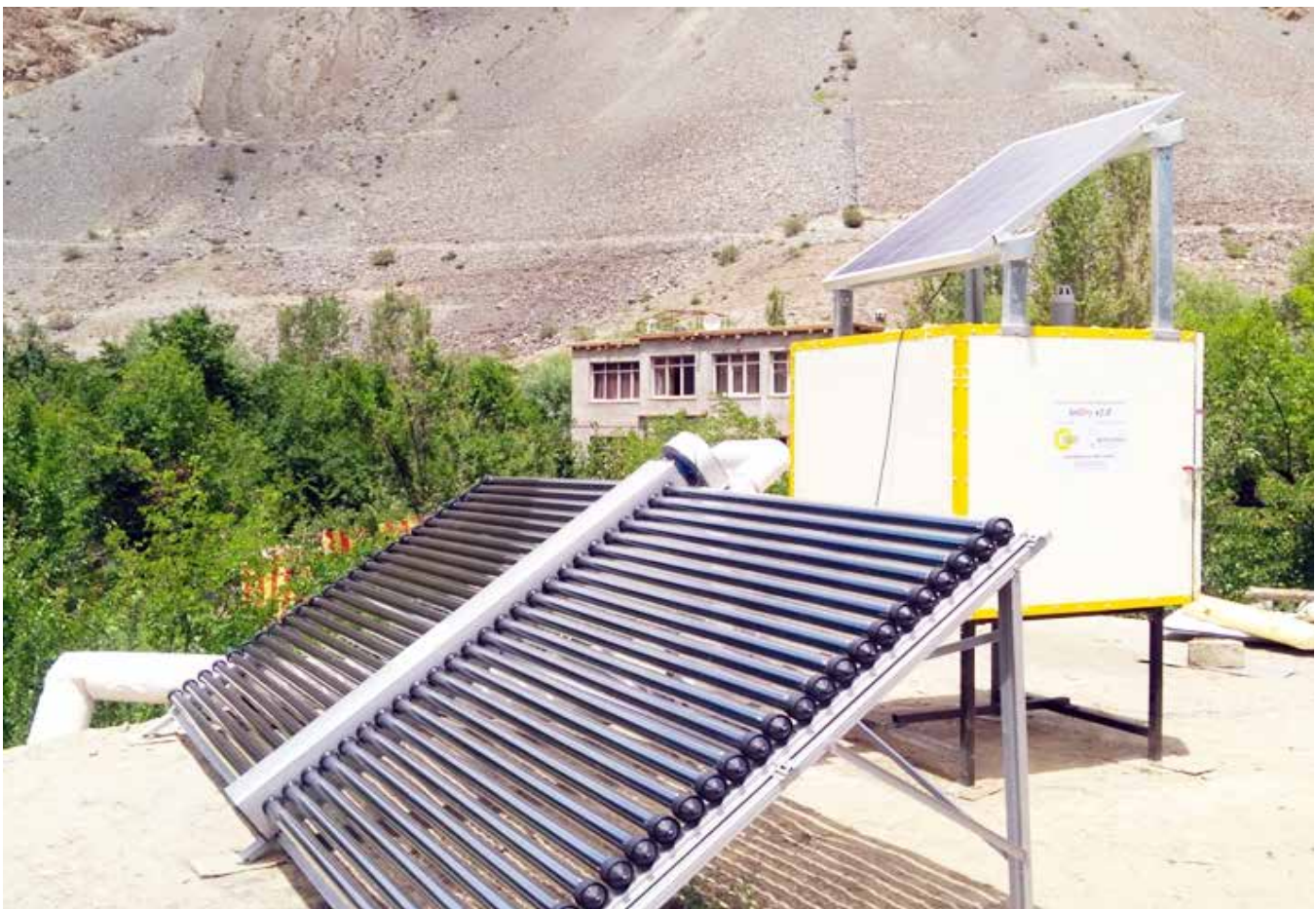
Figure 6.13: Solar Apricot Dryer Cum Space Heating System installed at Minjee Village, Kargil
