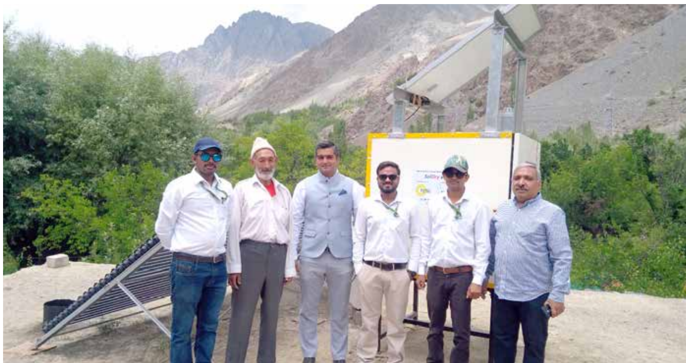
Figure 6.14: Solar Apricot Dryer Cum Space Heating System installed by NISE
