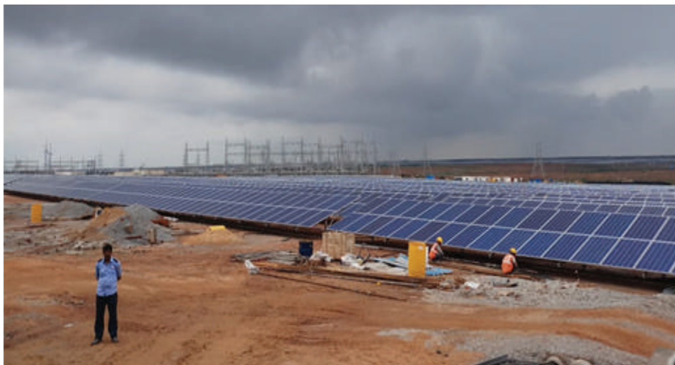
Figure 1.4. 750 MWp ultra mega solar power project at Rewa
