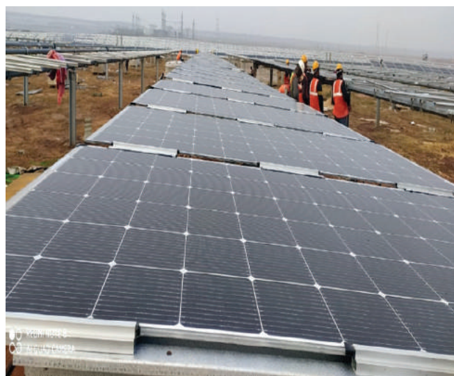
Figure 9.1. The 750 MW REWA Ultra Mega Solar project.
