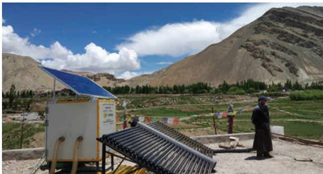
Figure. 7.11 Photograph of Solar Dryer cum Space Heating System installed in Ladakh
