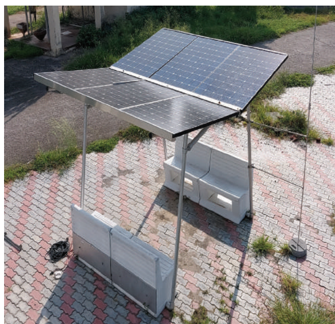
Figure 10.4: PV Port & Store System at NISE
