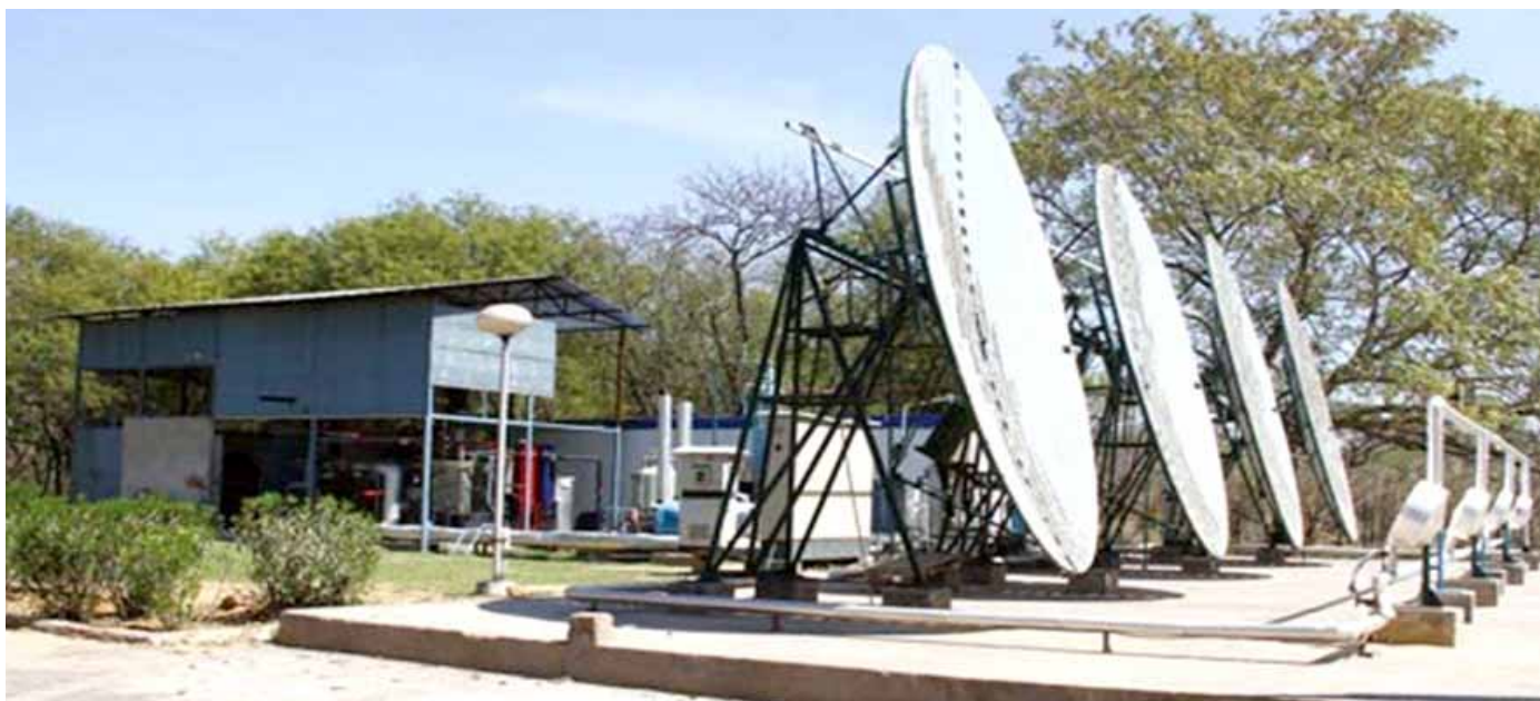
Solar Biomass System for electrification and cold storage
