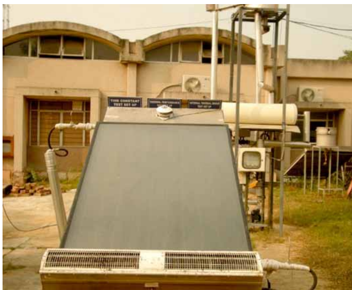
Testing of solar flat plate collector
