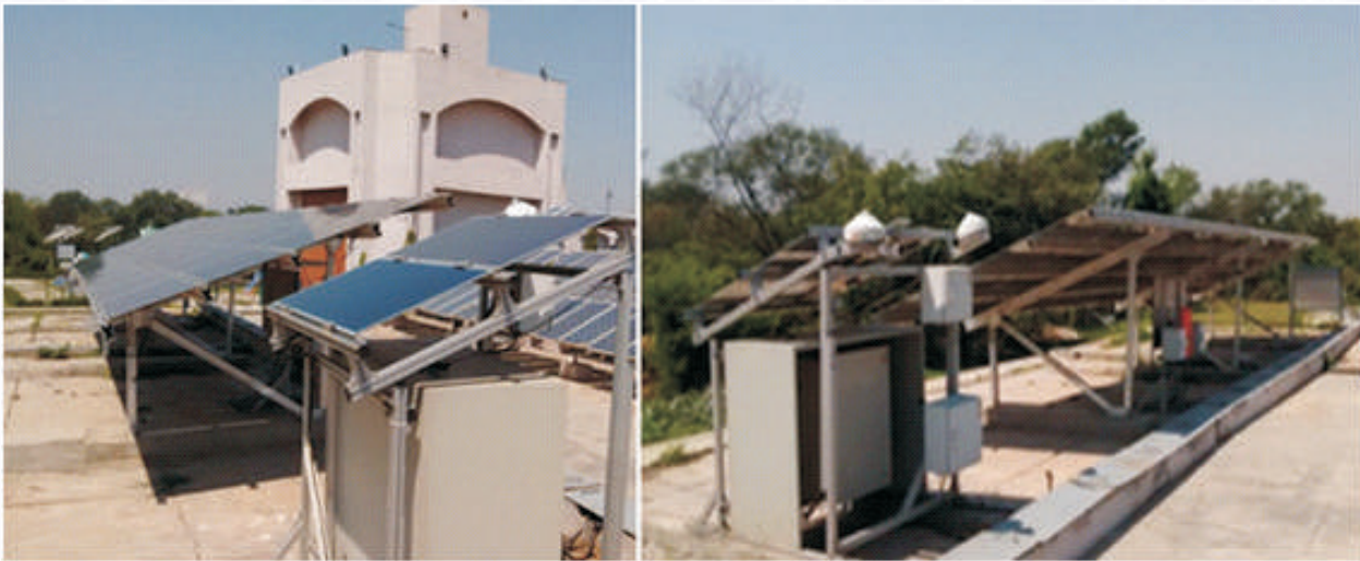
Fig. 3 Front and rear view of CdTe test bed installed at NISE
