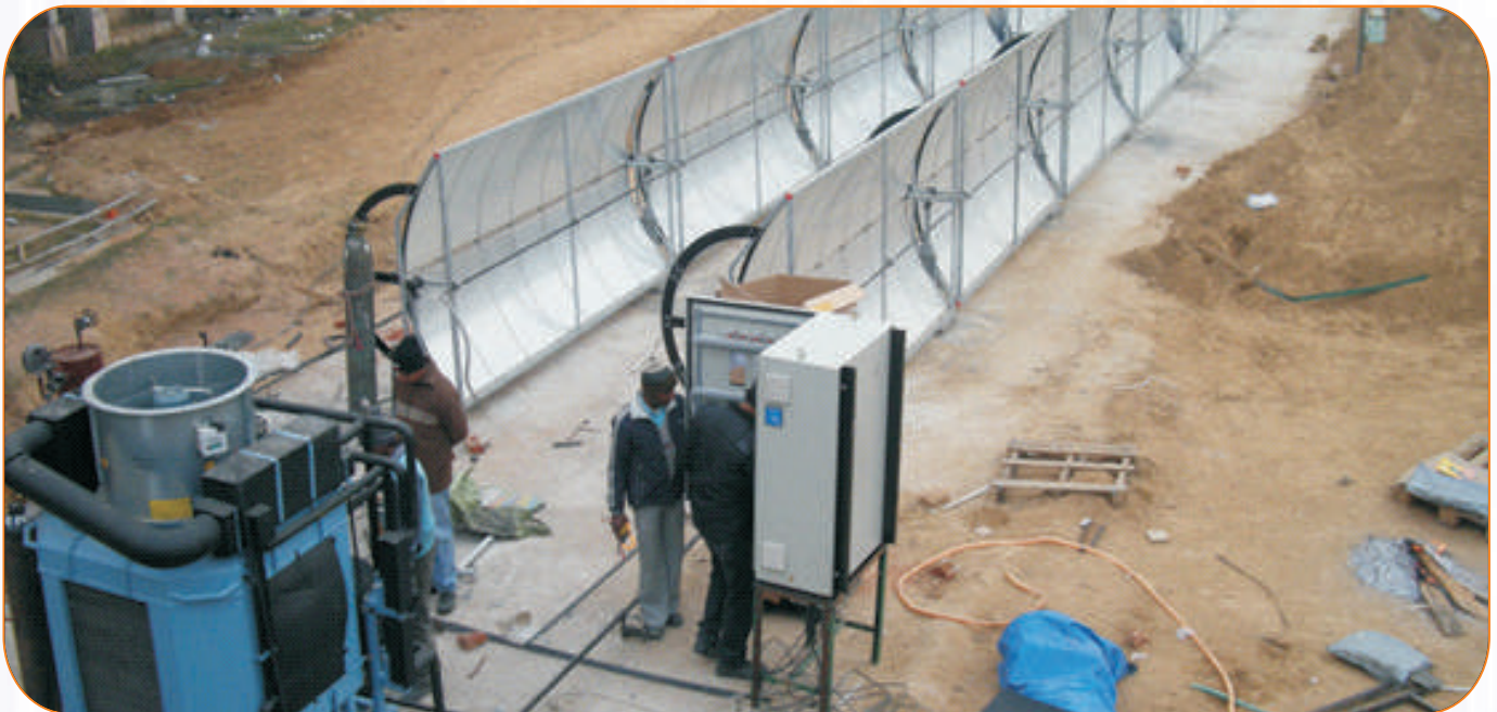
Fig. 3.6: 15 kW Solar Absorption Refrigeration System (Air Cooled)
