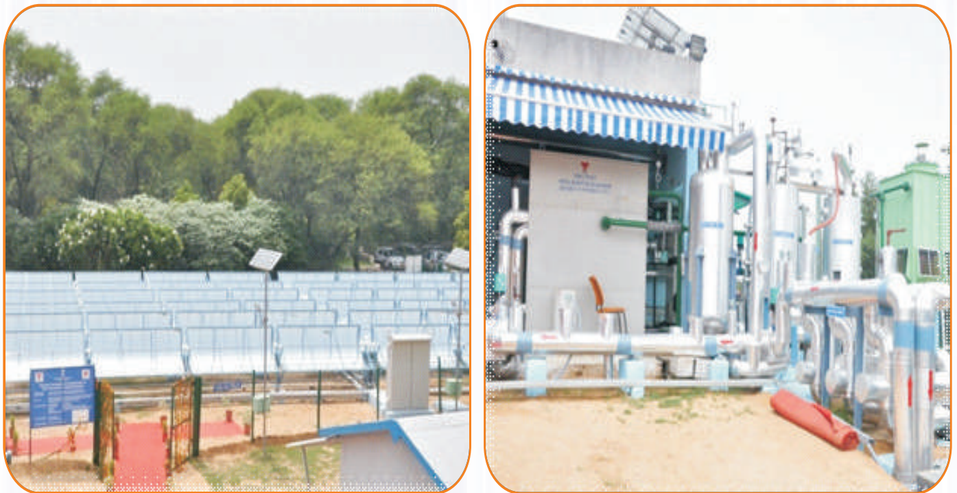
Fig. 3.4: Solar Field and vapour absorption machine
