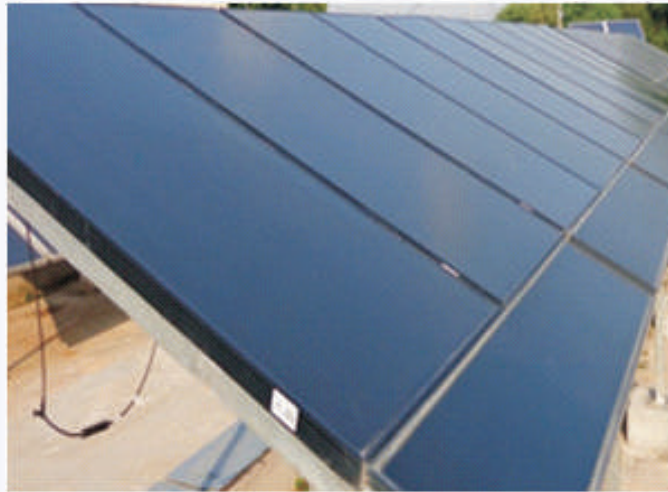
Fig.4 CIGS Test Bed Facility at NISE
