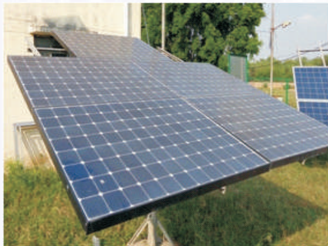
Fig. 5 Sun Power Array installed at the outdoor test bed facility of NISE
