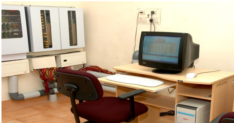
Fig.7. Photograph of data logging in solar station II
